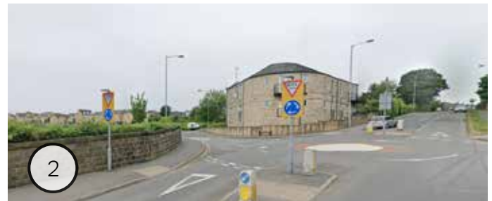
Poor pavement materials around a small roundabout at the junction of Warren Lane with Agincourt Drive and Rylands Ave;
