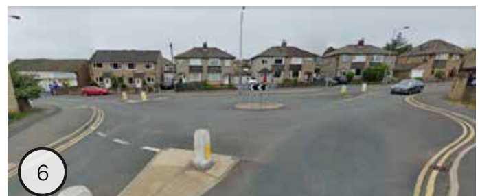
Poor pavement materials around a small roundabout at the junction of Warren Lane and Swan Ave;
